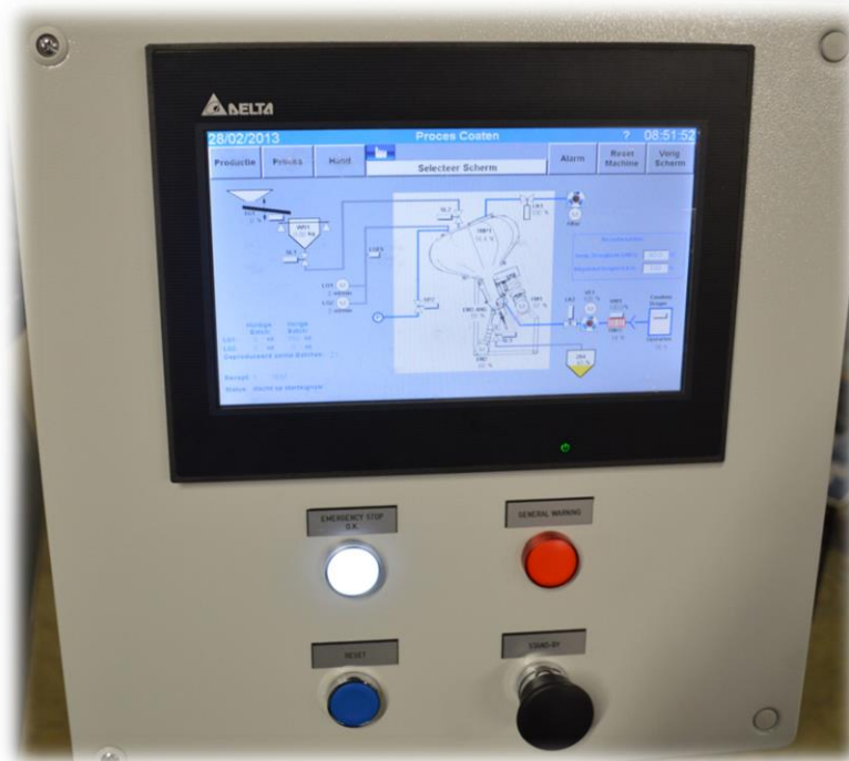
Complete process overview with 10" HMI
